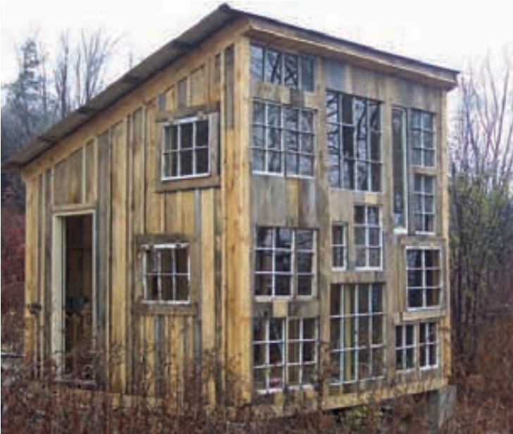
Twenty-five years ago, Andy Reichsman acquired 100 double-hung window sashes from a school that was replacing them. Today, some of those windows form the south wall of the cabin Andy built in Marlboro as an art studio for his daughter.
