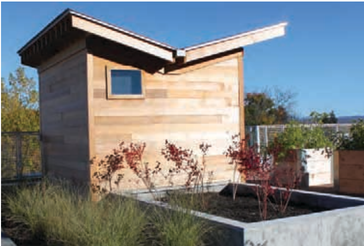
The H. Keith Wagner Partnership designed this water-harvesting shed as part of the new greenroof at Fletcher Allen Hospital. The V-shaped roof directs rainwater to holding tanks that can store up to 150 gallons; www.hkw-p.com .
